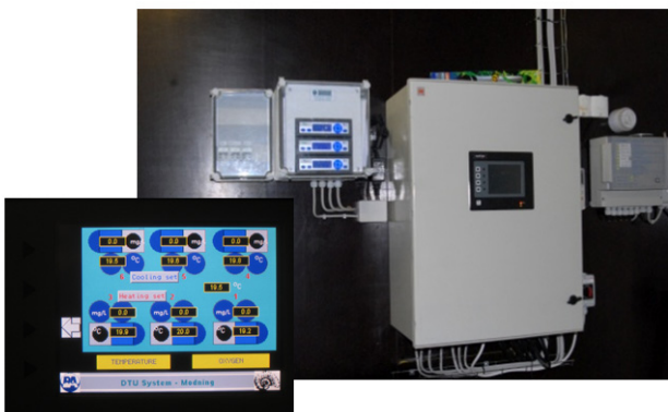
Figure 4.7.1. PLC system for registration and control of physical-chemical conditions in the recirculation systems
